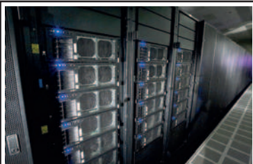
Part of the Roadrunner super-computer, built by IBM in 2008 for the U.S. Dept. of Energy
